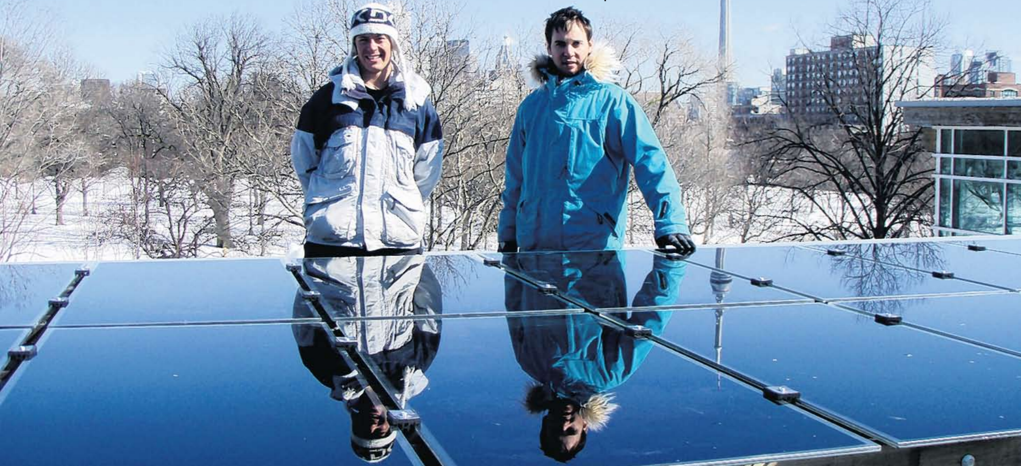
Global player: An EPOD installation given as a charitable donation to a community centre in Toronto, Canada
