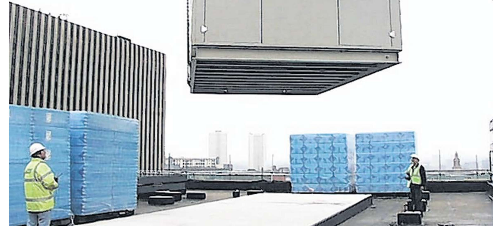
A Morgan Marine rooftop packaged substation
